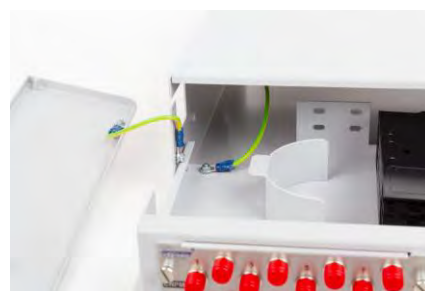
Detail of grounding
